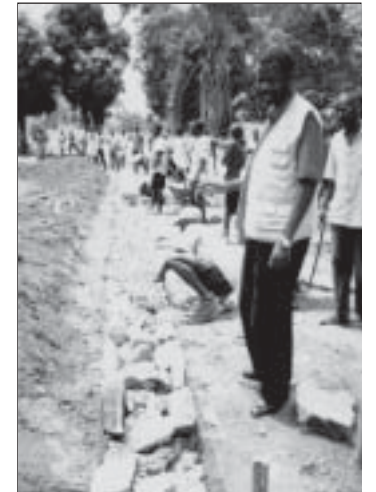
Rev. Andrew Mubugu Elisa at the construction site where a foundation is being laid for the facilities in Baguga.
